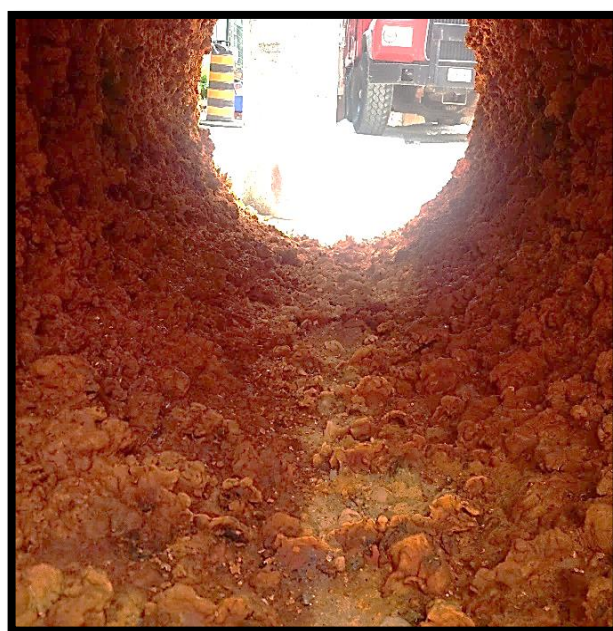
Section of old trunk watermain in Toronto, replaced in 2015.
